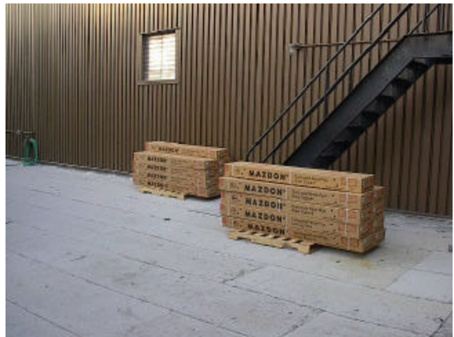
Figure 12: Tubes are delivered to the job site after pipe work is completed and system is switched to manual operation.
