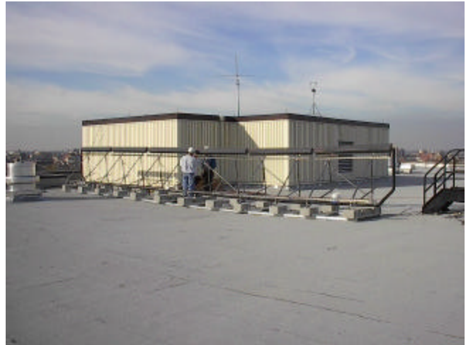
Figure 11: After all plumbing work is completed and leak test is conducted, vacuum tubes will be inserted.
